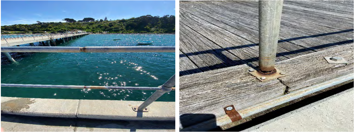
Figure 4-12: General condition of steel barrier (left) and localised failure at barrier connection (right)
