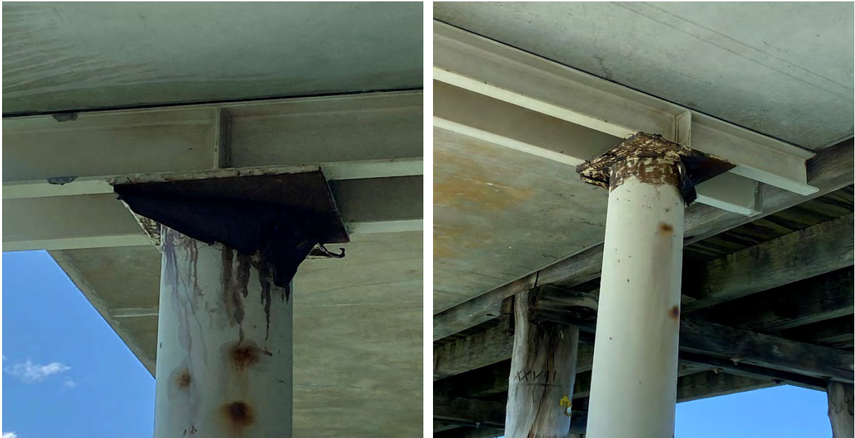
Figure 4-20: Material noted at top of steel piles and base plate location
