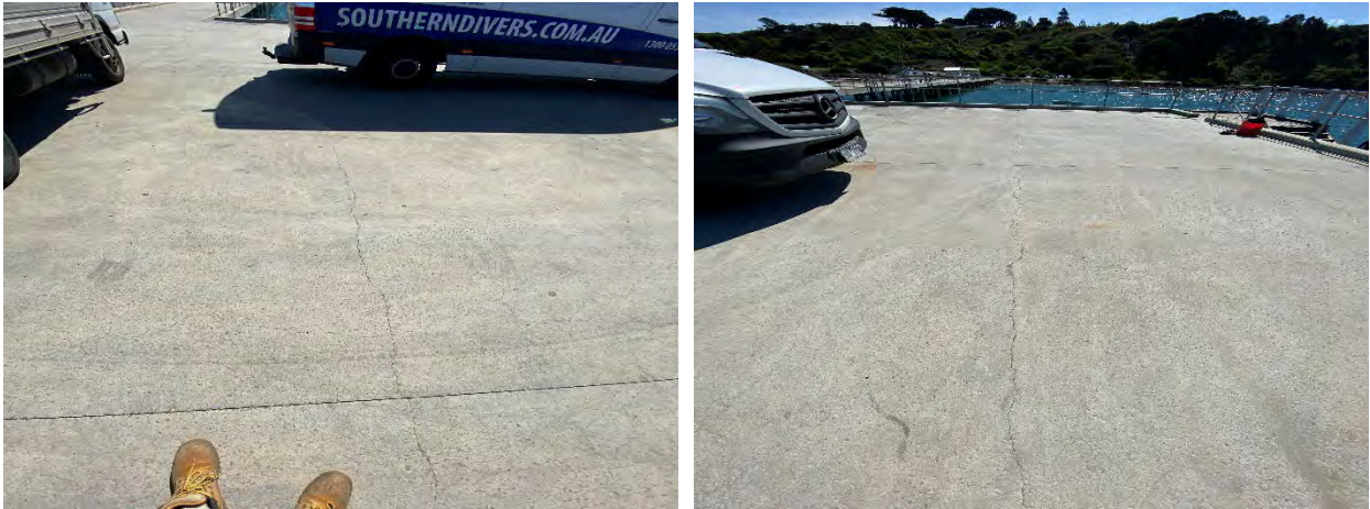
Figure 4-23: Longitudinal cracking in turning bay
