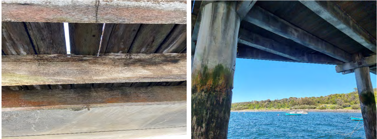
Figure 4-7: Top rot (left) and preventative membrane on newer members (right)
