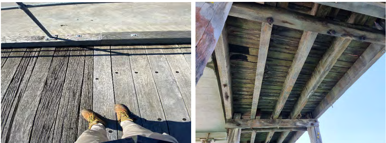
Figure 4-10: Comparison between new and older deck members (left) and localized fire damage (right)
