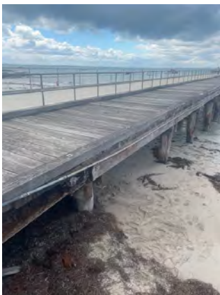
Decay and marine borers
