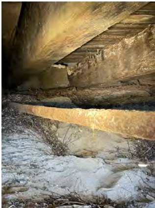
Ground contact of pier
