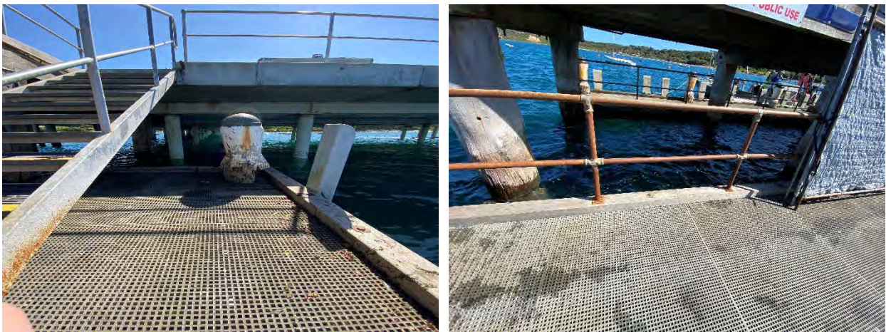
Figure 4-11: General condition of lower landing and barrier with corrosion
