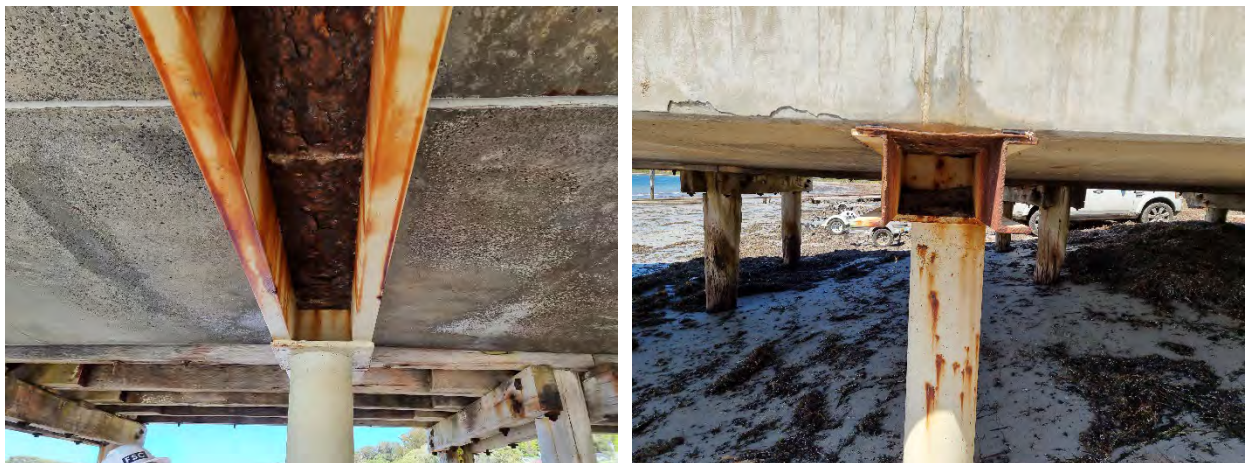
Figure 4-21: Rust staining of crossheads from plate above
