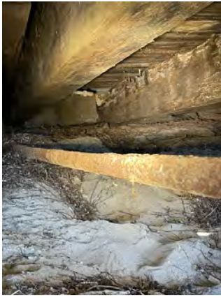
Damage to stringers attached to land
