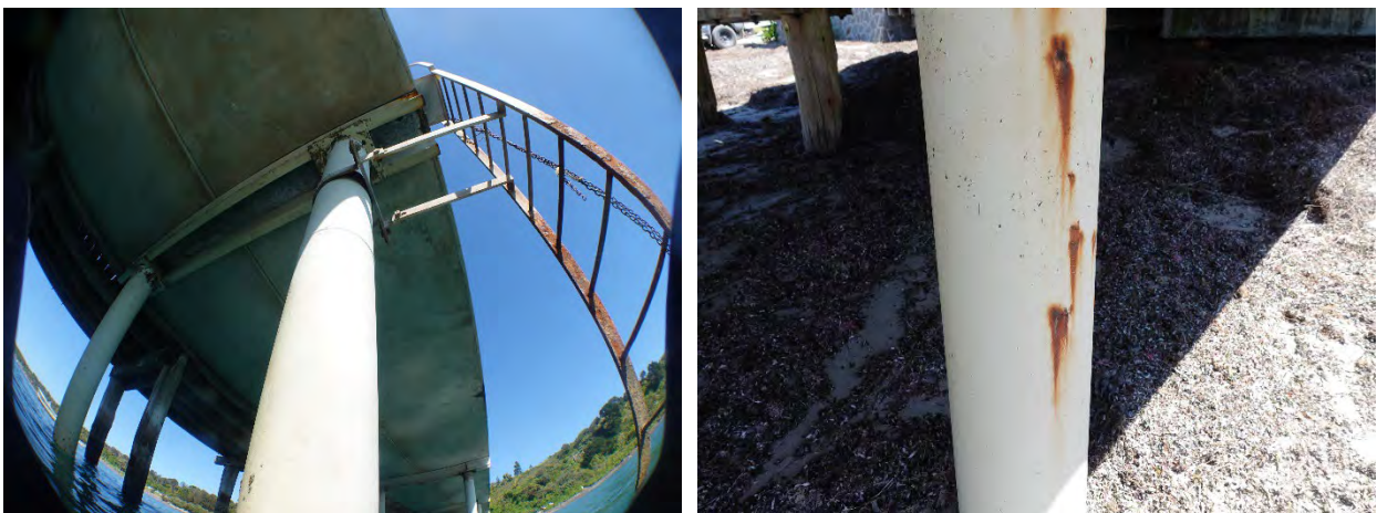
Figure 4-19: General condition of steel piles above water
