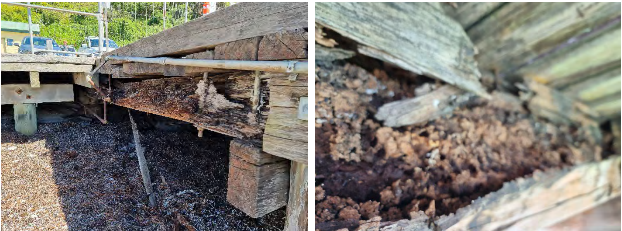
Figure 4-6: Beam 1E that has completely failed (left) and a close up view of termite attack (right)
