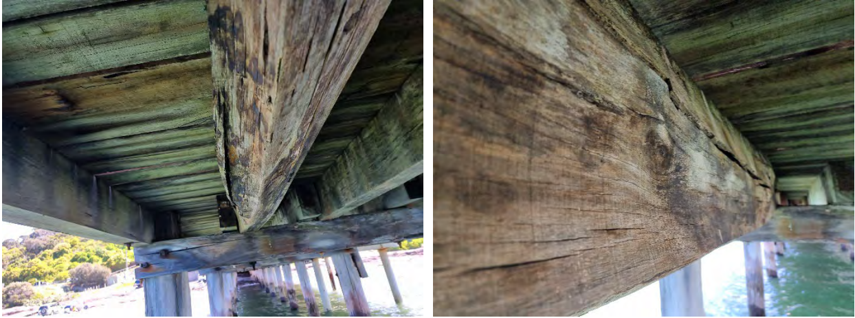
Figure 4-5: Hollowed out and crushed timber beams due to termite infestation
