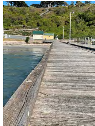
Sagging of pier 20-23c
