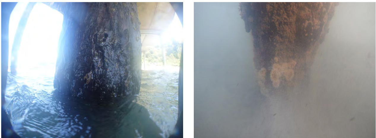
Figure 4-2: Pile 20B at the water line (left) and at seabed level (right)
