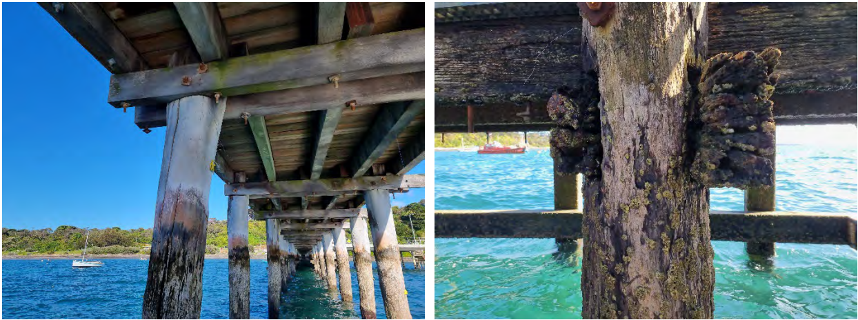
Figure 4-9: General condition of crossheads (left) and typical deterioration of member ends (right)
