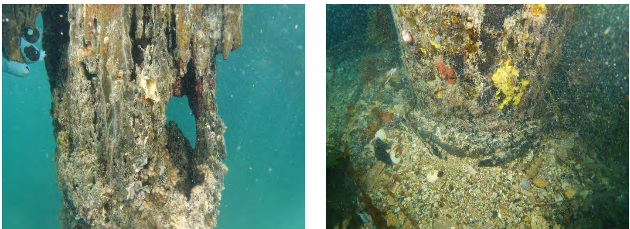
Figure 4-3: Localised cavity in Pile 44A (Condition 6 - left) and sound condition at seabed level (right)
